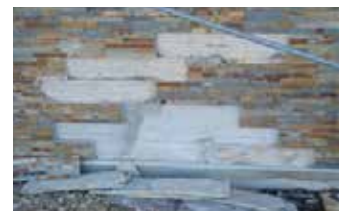
Delamination of Stone
